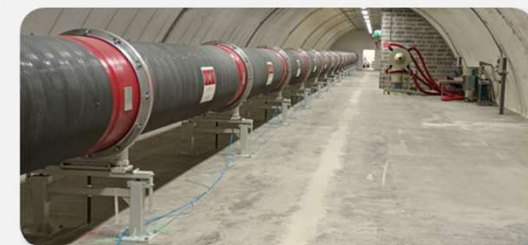
CICLoPE (Centre for International Cooperation in Long Pipe Experiments)
